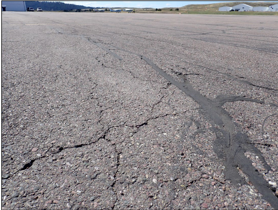
AP-11-34: Alligator Cracking
