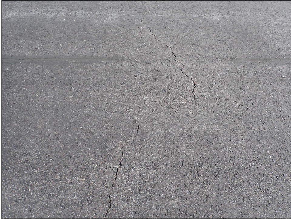
TW-11-26: L&T Cracking
